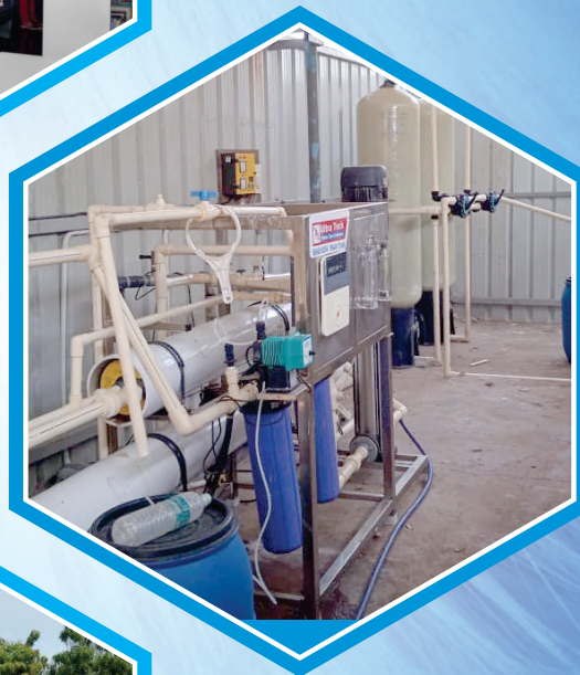
RO WATER FACILITY IN THE CAMPUS
