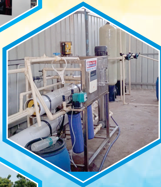
RO WATER FACILITY IN THE CAMPUS
